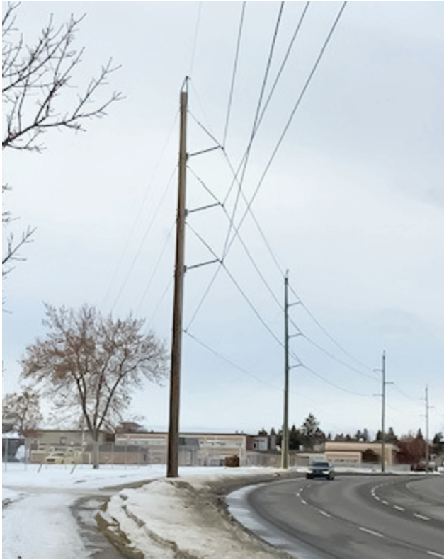
Example of Wood Pole
