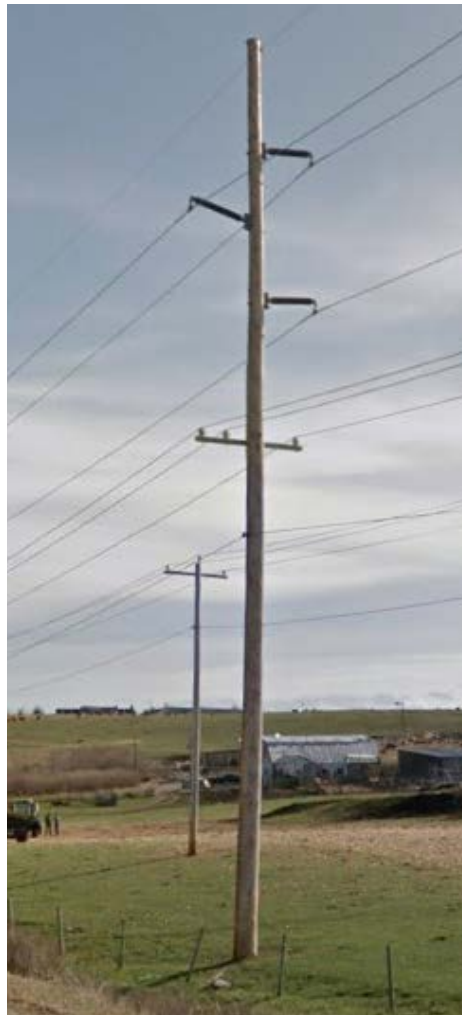
EXISTING WOOD POLE
