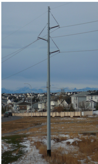
Example of Steel Monopole
